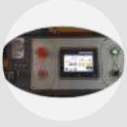
PLC Kontrol Panel PLC Control Panel
