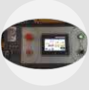
PLC Kontrol Panel PLC Control Panel
