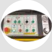
Kontrol Panel Control Panel
